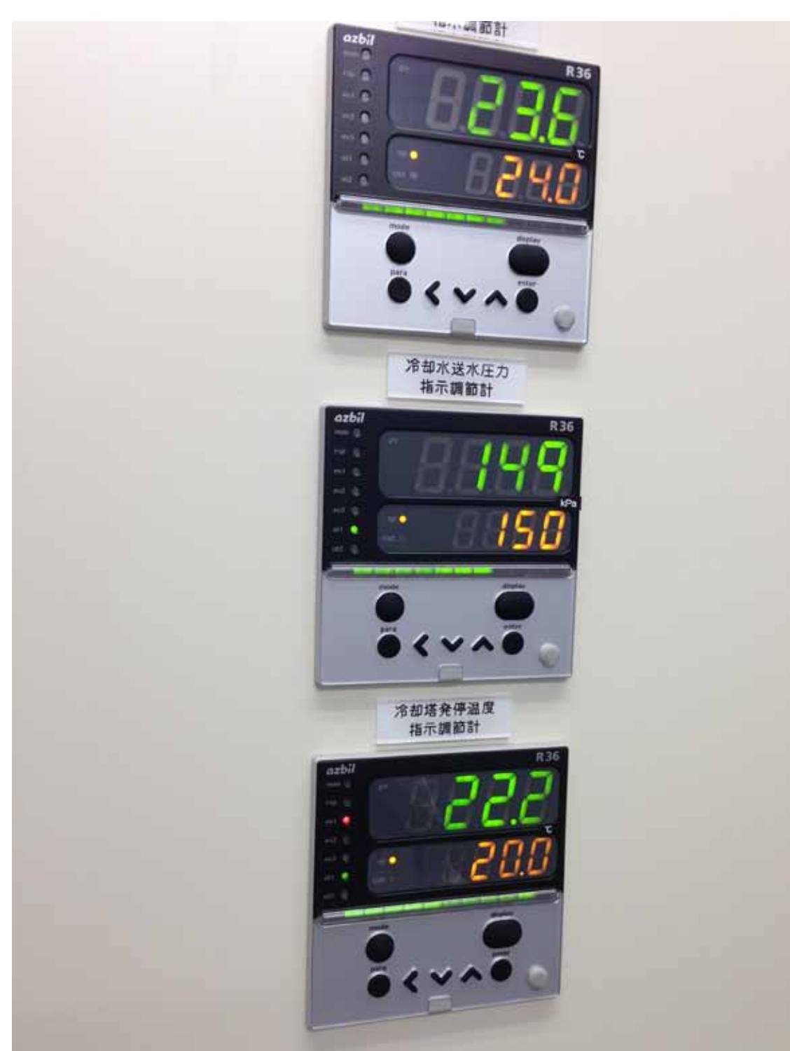
Control systems for cooling tower.
