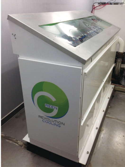
Fig. 3 The GRC Carnot Jet system installed inside the container
