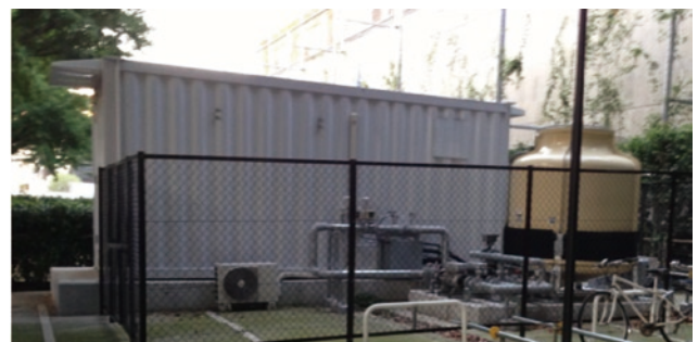
Fig. 2 Exterior view of TSUBAME-KFC: evaporative cooling tower right next to the 20-foot container for complete lights-out operation and low waterpump power
