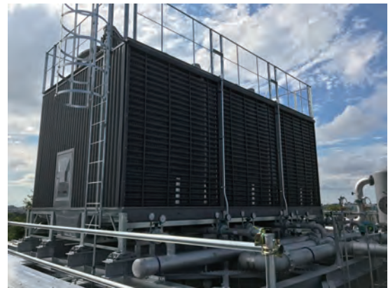
Cooling towers on the roof of the building
